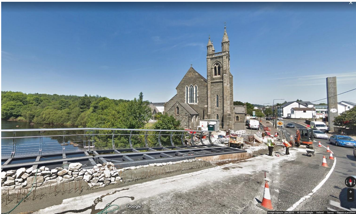
Plate 13-30: Reduction of parapet and widening of Ballybofey Bridge underway in 2018. Church of Mary Immaculate (Reg. No. 40838023) beyond (image from Google Street June 2018).
